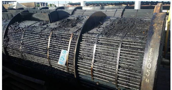
● Preheater train heat exchanger E-2505H decontaminated (0% LEL, 0% H 2 S, 0% benzene) using Vapour-Phase method in 11 hours without viscosity wash with LCO and Rezyd-HP Z71.*
