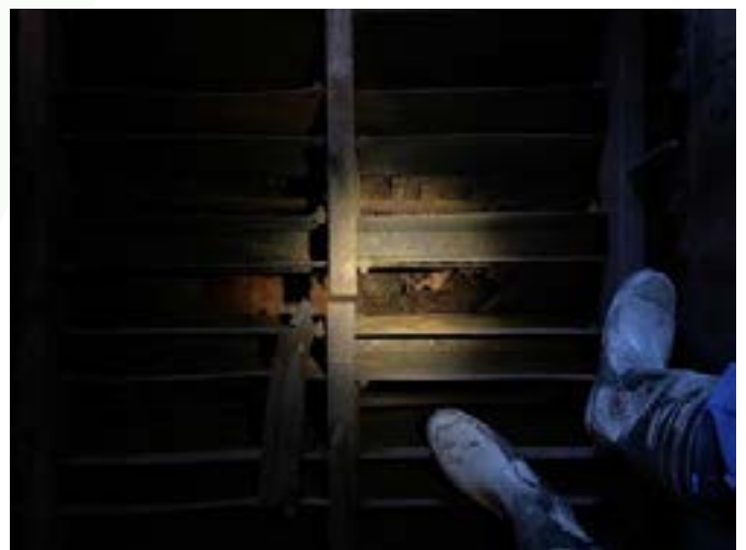
● DAMAGED PACKING BED FREE OF PYROPHORIC MATERIALS POST DECONTAMINATION
